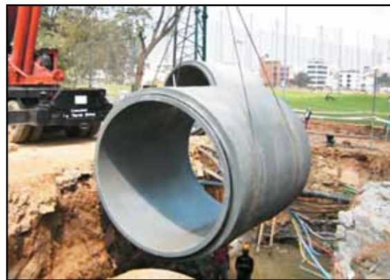
2400 mm dia R.C.C. NP-3 class pipe with polyurea lining for the sewerage work contract S2B for BWSSB, Bangalore
