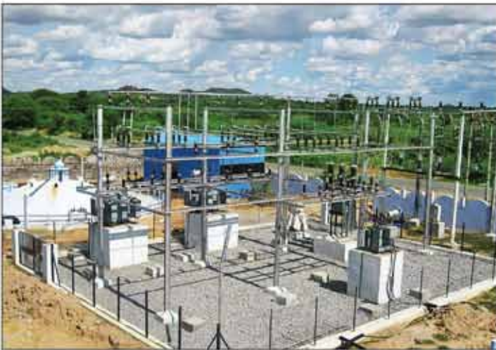
33 KV Sub Station
