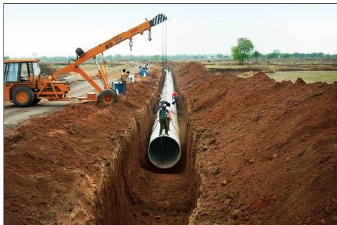
1700 mm and 1400 mm dia M.S. Pipeline for Raipur Augmentation Water Supply Scheme.
